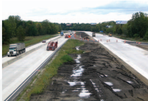
SDA's 2006 design of the I-94 Concrete Overlay in St. Clair County received the Michigan Concrete Paving Association's (MCPA) award for Overlay Project of the Year.
