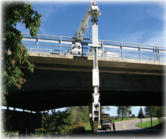
The Snooper Bridge Inspection Crane was utilized on the Huron Parkway Bridge Rehabilitation Project and the 2006/2007 Bridge Inspection Program.
